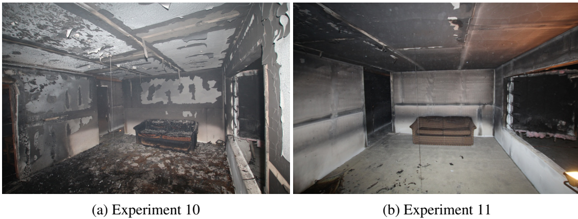
Figure 6.36: Post-suppression comparison of living room wall remote from kitchen with open door.
