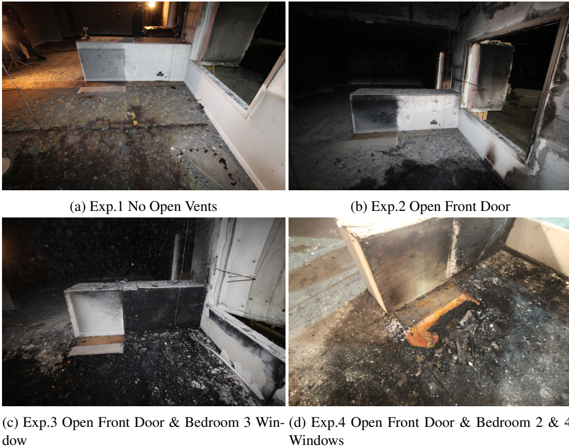
Figure 6.102: Experiments 1–4, fire damage in the family room TV area after removal of furniture.
