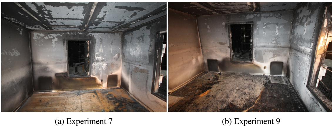
Figure 6.43: Post-furniture removal comparison of bedroom 1 area of origin with closed door and windows.
